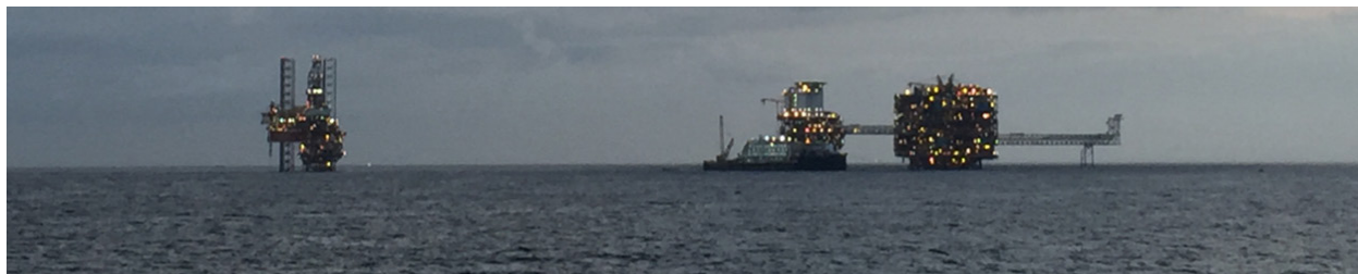
Figure 9. A drill rig attached to a completed wellhead platform on left; production complex under construction on the right
